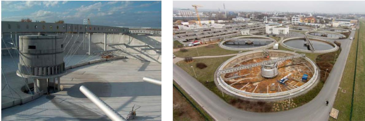
Figure 9: Secondary clarifier of the Dresden-Kaditz wastewater treatment plant. Left: existing, right: during modification.
