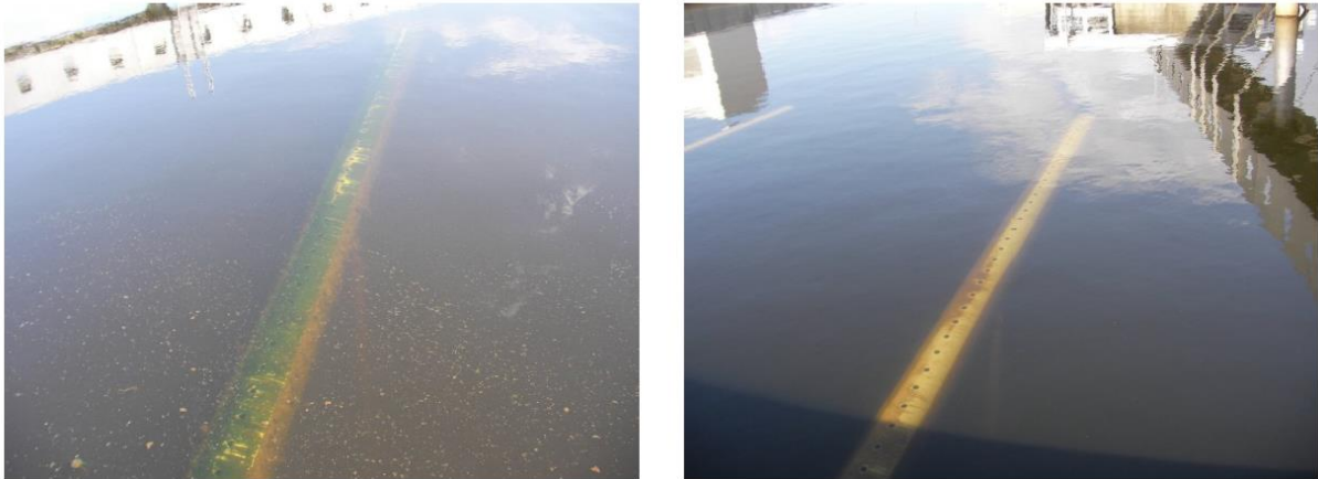
Figure 12: Photos from May 2015 of the secondary clarifiers in the area of the drain pipes in a tank with a rigid inlet structure (left) and an already modified tank (right).
