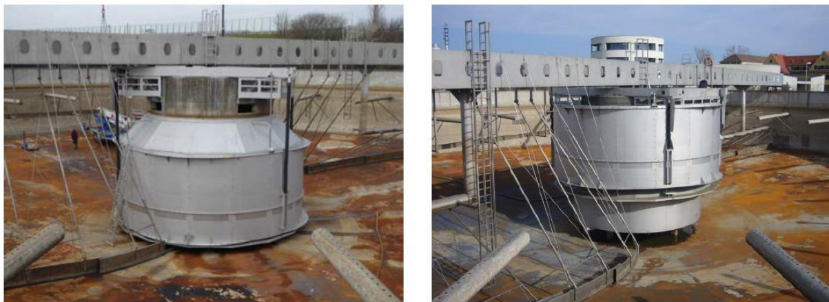
Figure 10: Height-variable inlet Passavant® hydrograv® adapt System in a secondary clarifier of the Dresden-Kaditz wastewater treatment plant. Left: in low position, right: in upper position.
